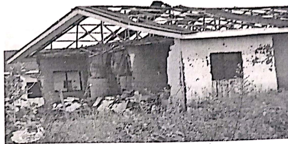
Plate 2: Collapse building due to weak materials and poor construction
