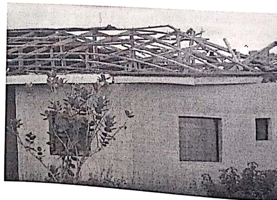
Plate 1: Roof of a building affected by the rain/wind storm
