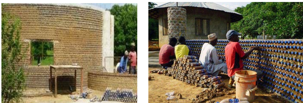
Fig. 1&2: Nigeria's first house built from discarded plastic bottles under construction. Source: globalwasteideas.org (2015)
