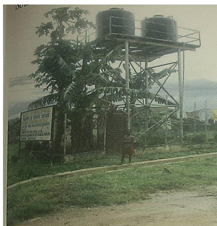
Plate 3: Public Solar-Powered Borehole with Overhead Water Tank in Ibulesoro
