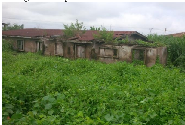
Figure 5: Flooding and Corrosion Effects on Residential Property at Isolo Quarters, Akure
