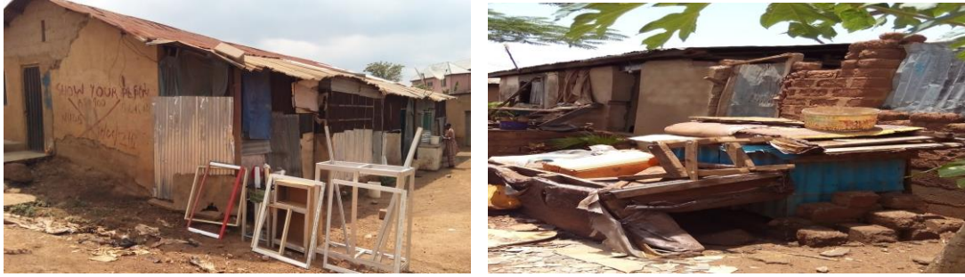
Plate 11&12: Structural Quality of Houses in the study area
