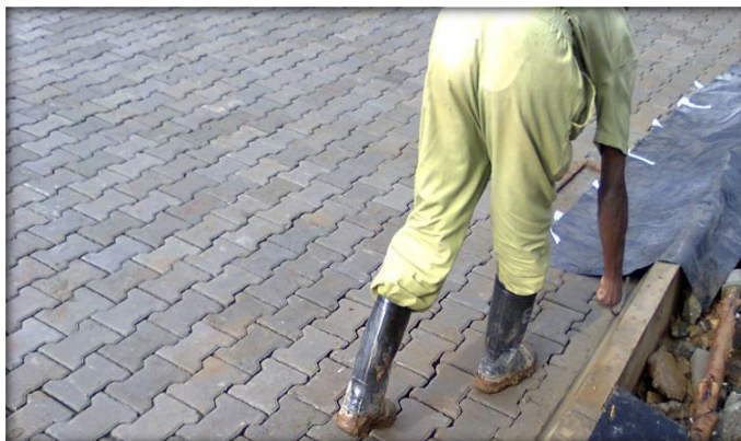
Figure 2 - Polythene cover was placed after placing mortar between kerbstone and paver block
