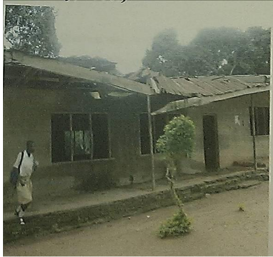
Plate 1: A dilapidated secondary school building at Ibulesoro
