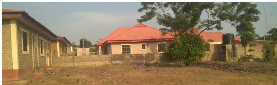
Fig. 4: Picture showing open space at back of a building transformed to another building using sandcrete blocks
