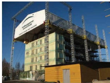
Fig. 2: Eight-Story Building under Construction Protected with a Tent in Sweden (Source; Mohammad et al. , 2015)
