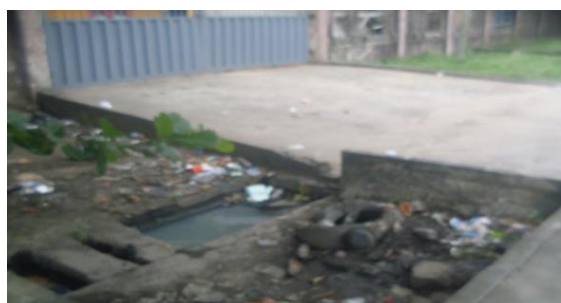
Figure 7: Poor drainage in off Bishop Oluwole Street, Victoria Island in Eti-osa
