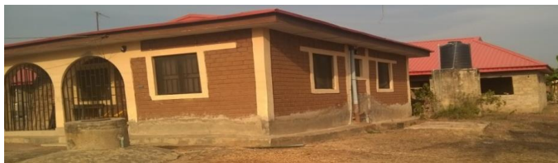
Fig. 3: Picture showing proper ventilation of the buildings
