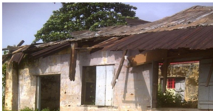
Figure 3: The existing schools in the community are in a state of disrepair
