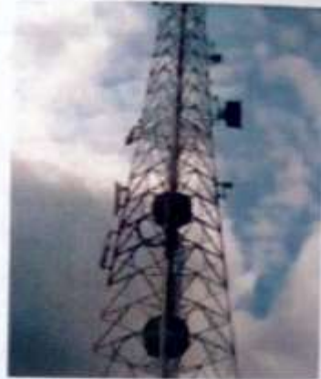
Fig 6: GSM Mast with micro wave and sector antennas mounted typically found in a BSC/BTS site
