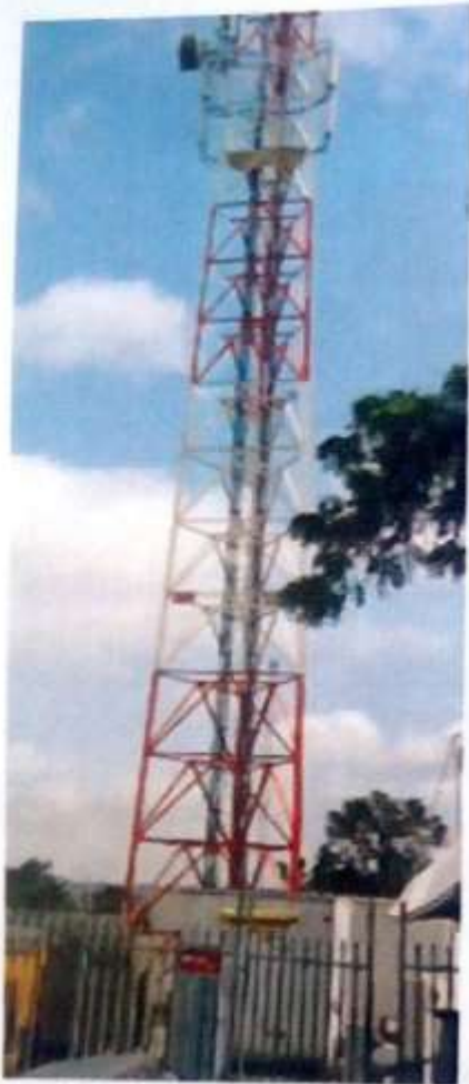
Fig 5: BTS site with mast view
