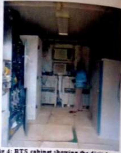
Fig 4: BTS cabinet showing the digital equipment, air conditioner, and power unit.
