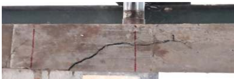
Figure 4b. Failed beam
