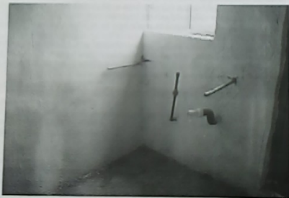
Plate I: Vandalized Fittings in the Housing Unit Source: Field Survey, July 2010
