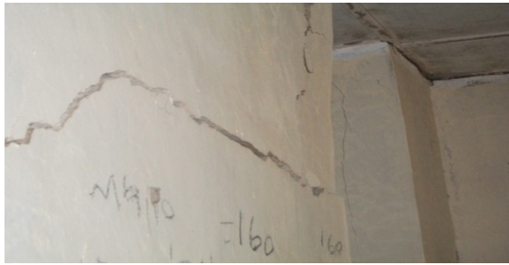
Fig. I. Hollow Block Wall Failure
