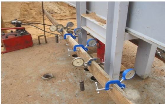
Fig. 5: Dial gauges for Settlement Reading
