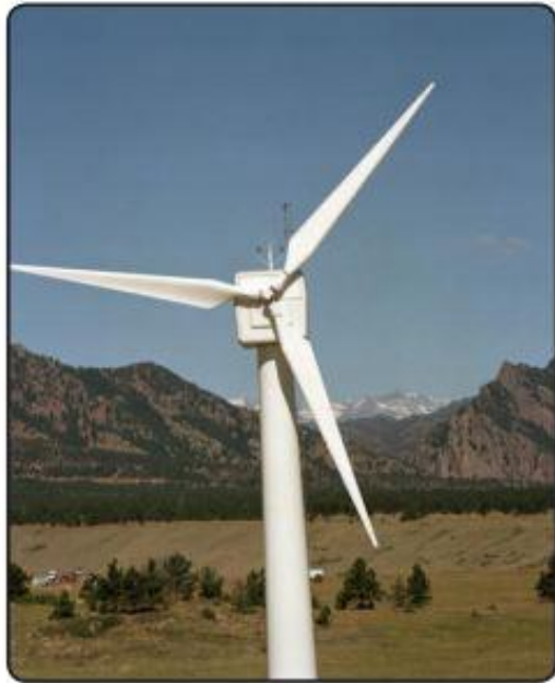
Figure 10: Horizontal Axis Wind Turbine. Source (Patel, 1999)
