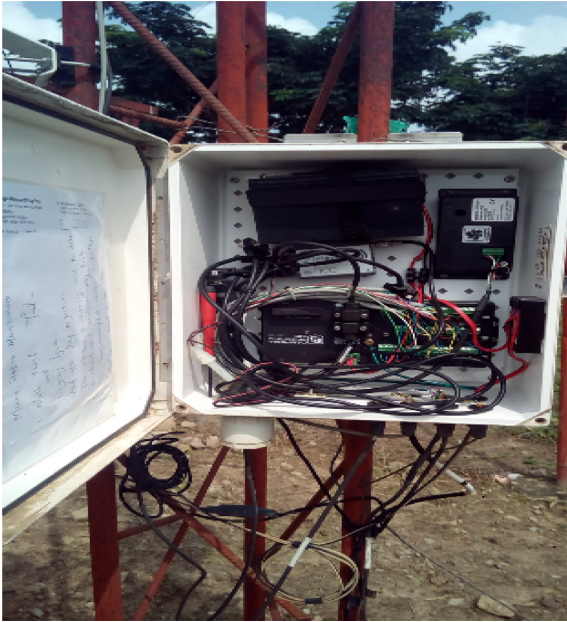
Fig. 2. Campbell CR-1000 data logger.
