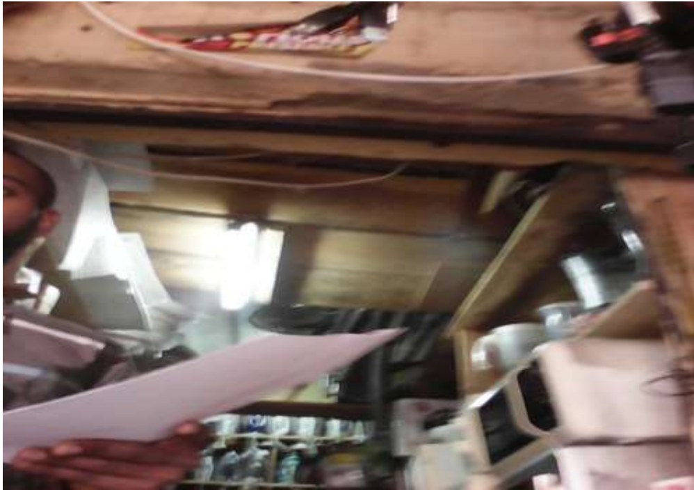
Plate LII: Non-fire resistant wooden ceiling in a lock-up shop in the central part of Wuse market. Source: Field work (2017).
