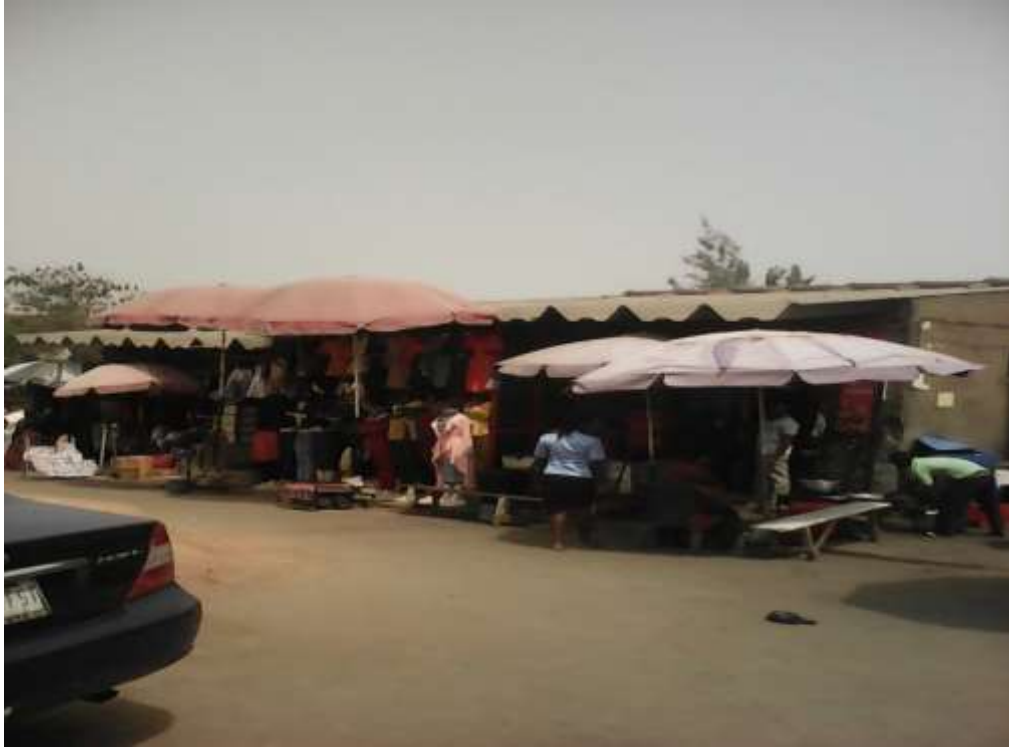
Plate LVI: Building with non-fire resistant asbestos roofing sheets in the southern part of the formal section of Garki model market. Source: Field work (2017).
