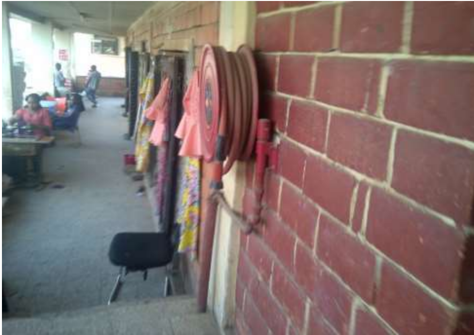
Plate LXI: Non-functioning fire hose reel at the ground floor level of a shop building in the northern part of the new section of Wuse market. Source: Field work (2017).
