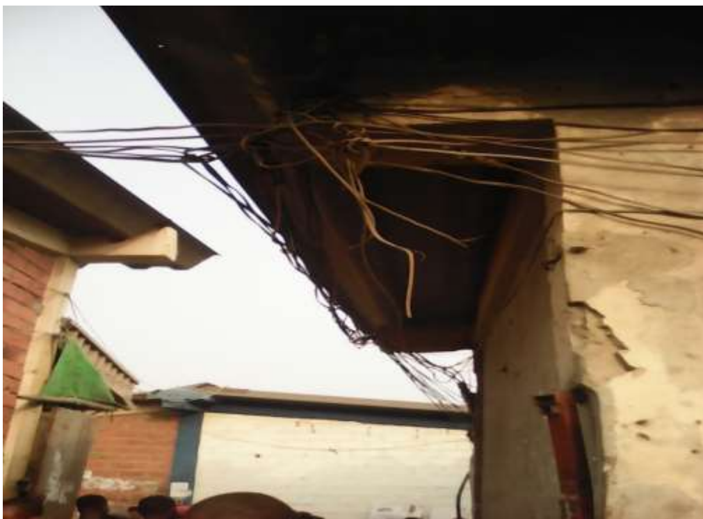
Plate XXIX: Illegal electrical connection at the eave of a roof in the central part of Wuse market. Source: Field work (2017).
