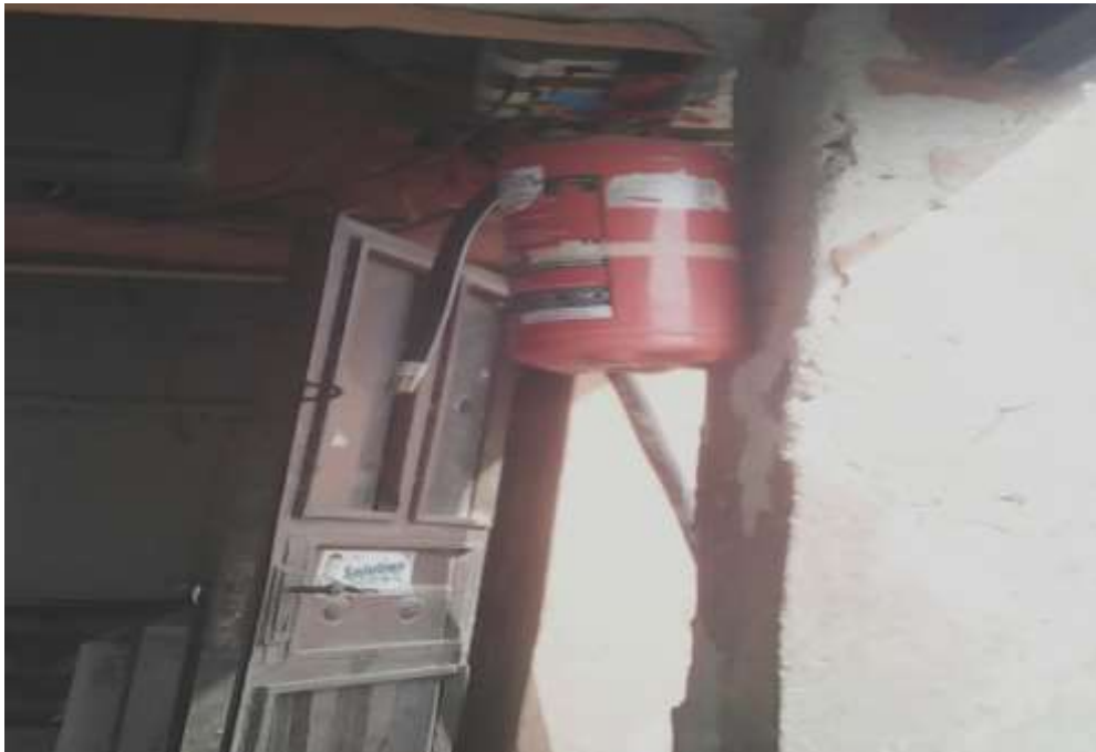
Plate LXIV: Portable extinguisher for fire which is attached to the front wall of a lock-up shop building in the central part of Kado market. Source: Field work (2017).
