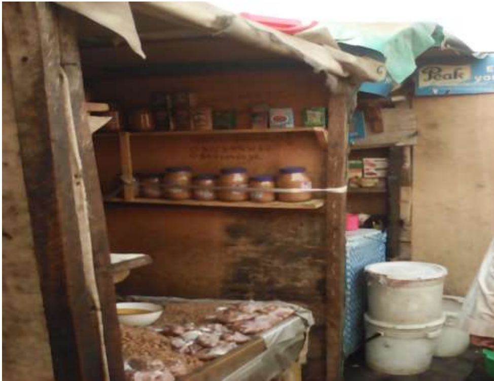
Plate XX: Erection of illegal non-fire resistant wooden structure for food stuff shop with zinc and tarpaulin roof coverings in the northern part of the old section of Wuse market. Source: Field work (2017).
