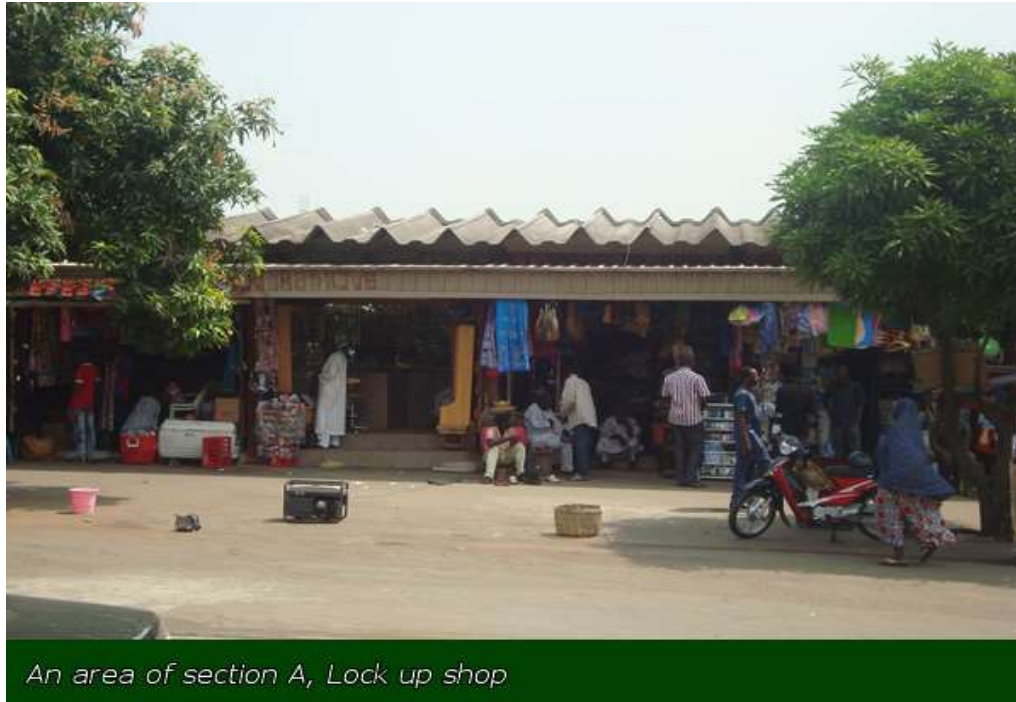
Plate XVI: Overcrowded nature of lock-up shops with non-fire resistant aluminium roofing sheets as sun shading device for corridor in Wuse market. Source: Abuja markets management limited, 2016 ( http://www.abujamarketsmanagement.com/wuse-market/ ).
