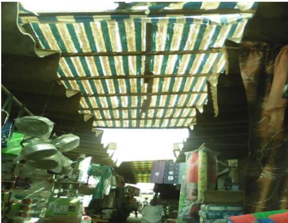
Plate XXV: One of the roof canopies as a shading device for sun in Garki model market. Source: Field work (2017).
