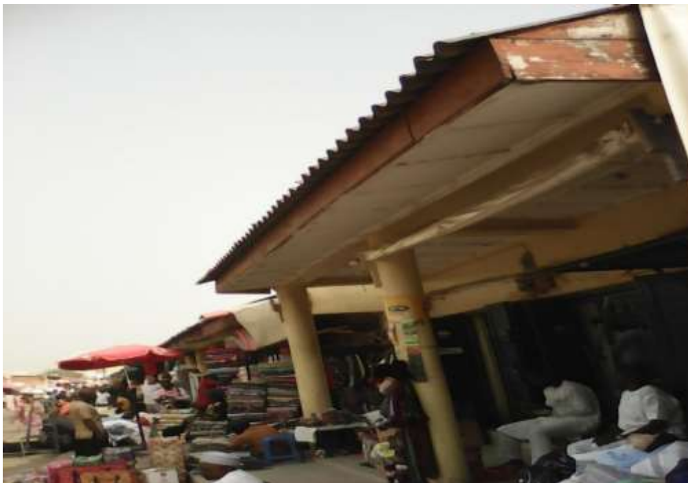
Plate LIX: Non-fire resistant wooden fascia of a lock-up shop building in the central part of the old section of Wuse market (source: field work, 2017).
