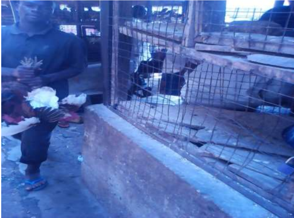
Plate XXIV: Non-fire resistant wooden fowl cage in the informal section of Garki model market. Source: Field work (2017).
