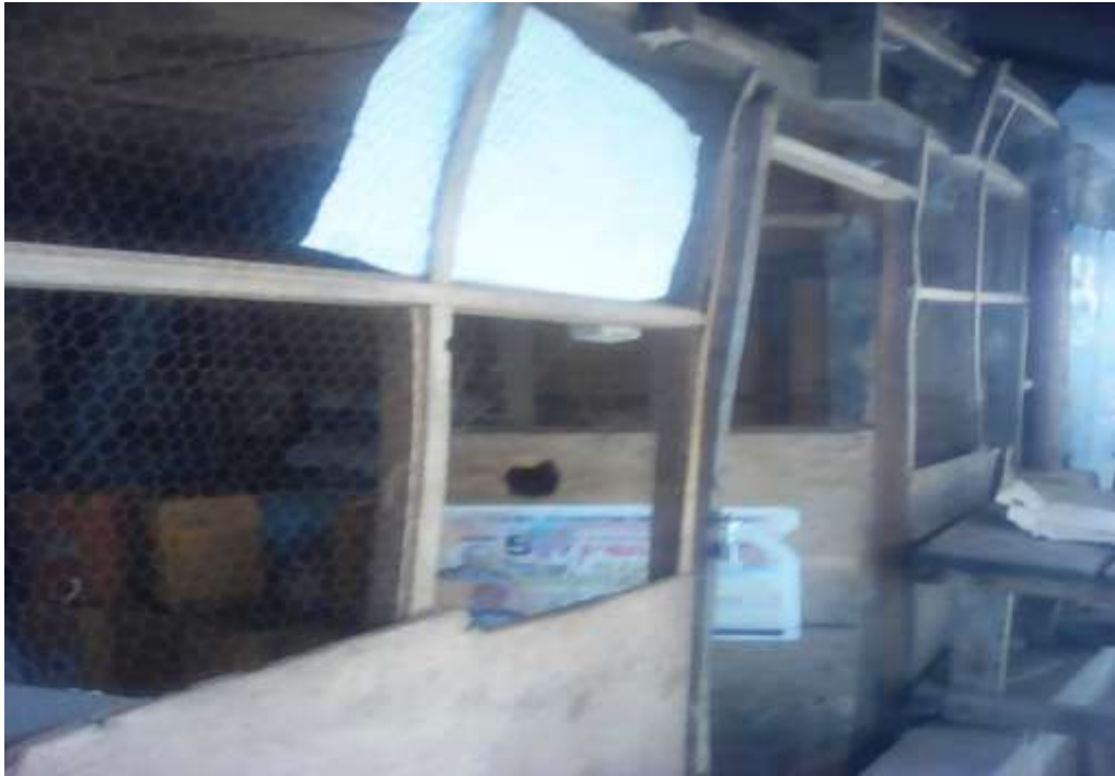
Plate XXVI: Non-fire resistant wooden attachment to a store building around the cold room section in the eastern part of Kado market. Source: Field work (2017).
