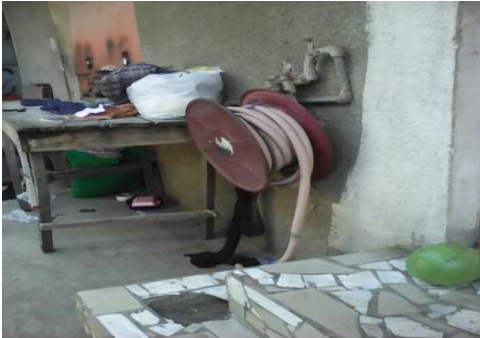
Plate LXIII: Non-functioning fire hose reel in the central part of the formal section of Garki model market. Source: Field work (2017).
