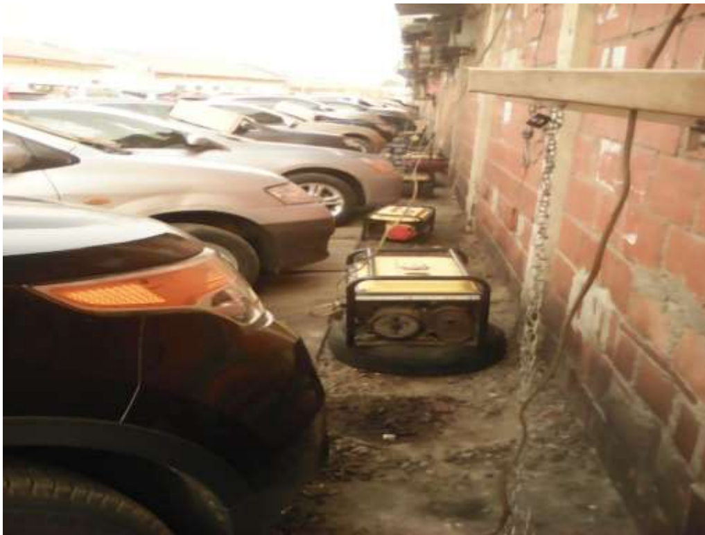
Plate XXXIII: Parking of cars close to the electric power generators that are working with petrol at the back of a lock-up shop building in the eastern part of the old section of Wuse market. Source: Field work (2017).
