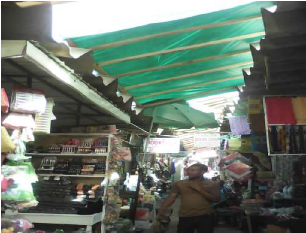
Plate LX: Non-fire resistant aluminium fascia of a lock-up shop building in the formal section of Garki model market. Source: Field work (2017).
