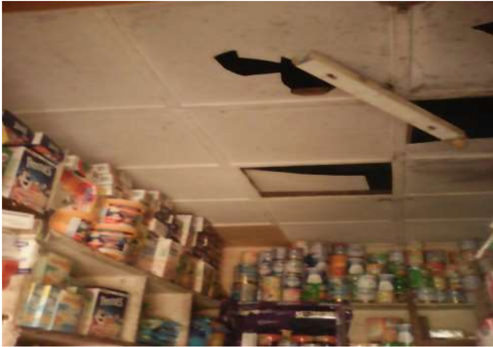
Plate LIII: Non-fire resistant asbestos ceiling board in a provision shop in the central part of the formal section of Garki model market. Source: Field work (2017).
