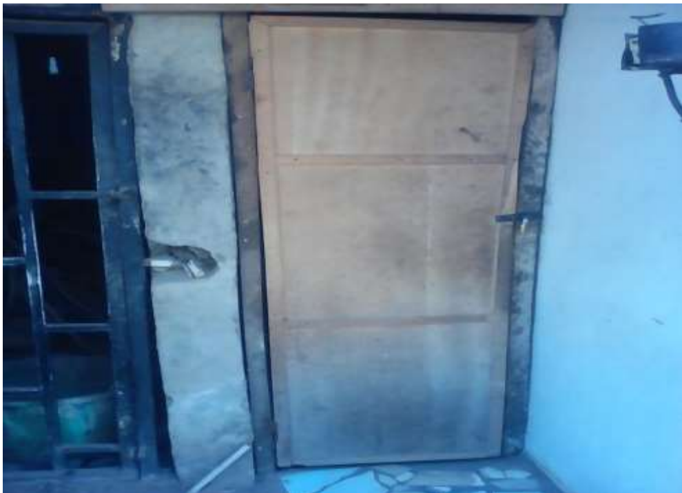
Plate LI: Non-fire resistant wooden door of a store building in the eastern part of Kado market. Source: Field work (2017).
