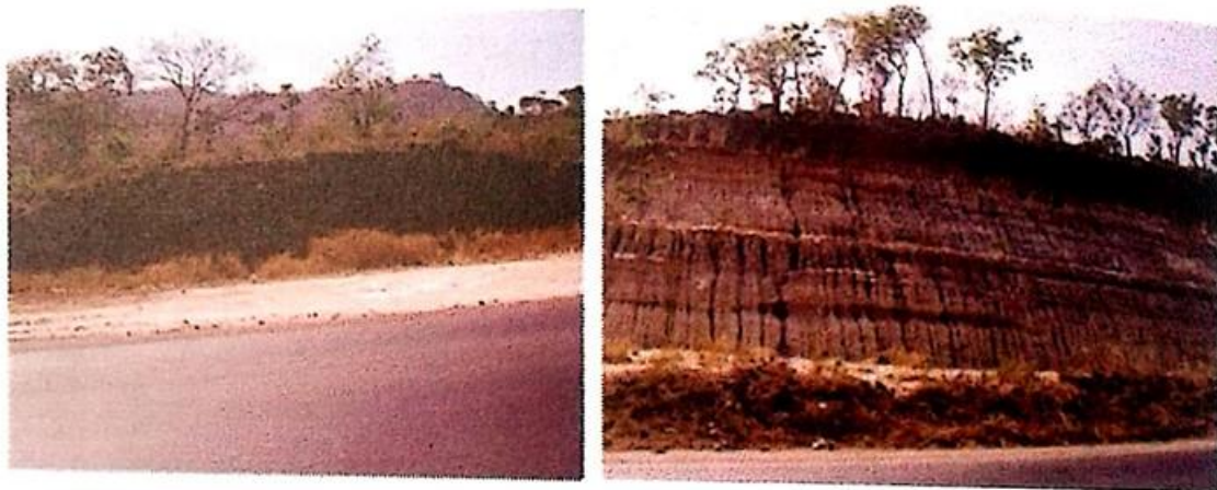
Fig. 14. Basal conglomerates (0) and poorly sorted muddy sandstones of the Lokoja Formation exposed 1 Km from the Lokoja-NATACO junction on the Lokoja - Abuja expressway
