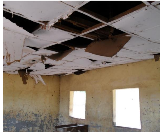
Plate 5: A dilapidated ceiling of one top primary school in Rafin Gora
