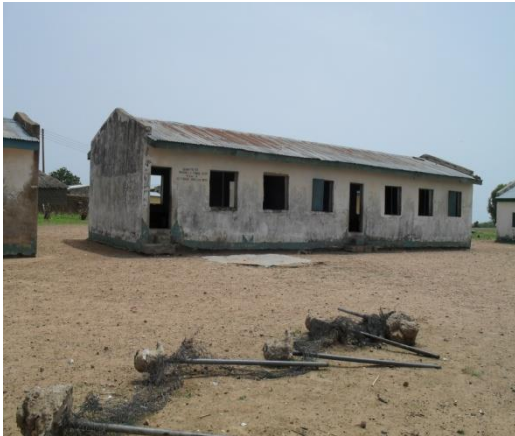
Plate 4: A dilapidated primary school in Tugan Magagiya
