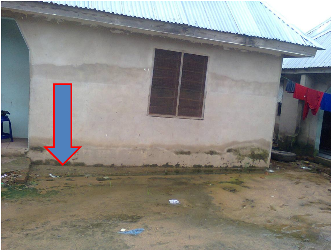
Fig. V: imprint of flood on building’s wall, signifying the level or height of flood waters at the time of impact. (Source fieldwork)
