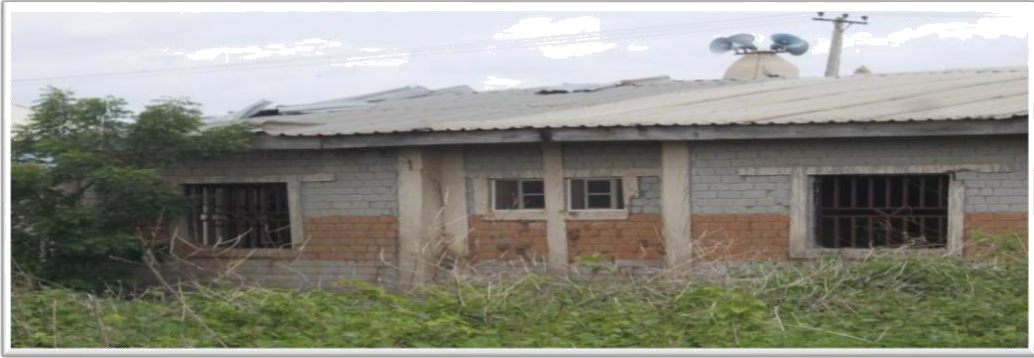
Plate V: A building showing windows removed at Harmony estate
