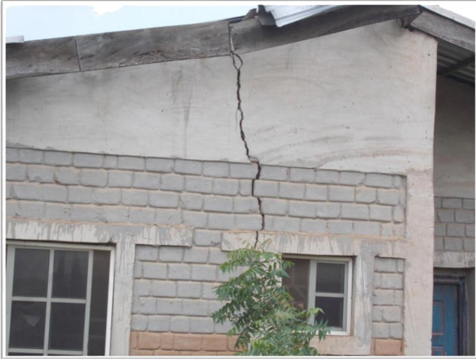
Plate I: Cracked wall of a building at Mandate housing estate
