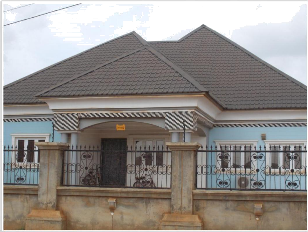
Plate IV: A building showing the good condition of roof at Royal valley estate
