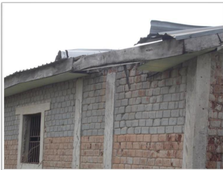
Plate III: A building showing some parts of the roofs missing at Mandate estate
