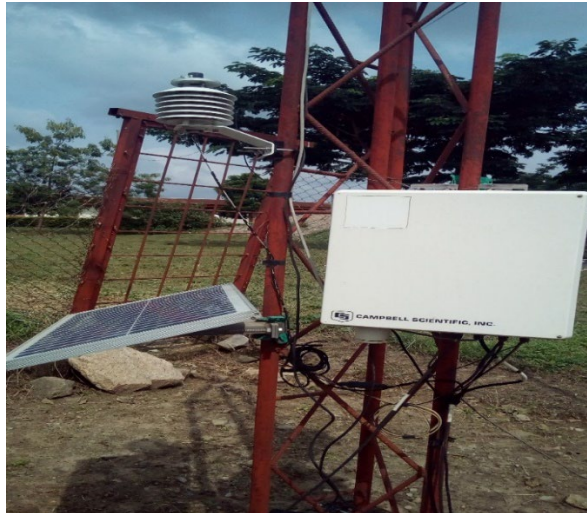
Fig. 2 - TRODAN weather station with Campbell CR-1000 data logger inset
