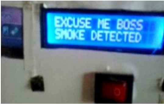
Figure 7: implemented system showing smoke detected
