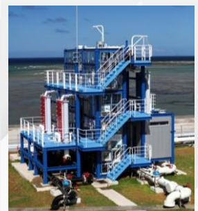
On-land OTEC Pilot Plant
