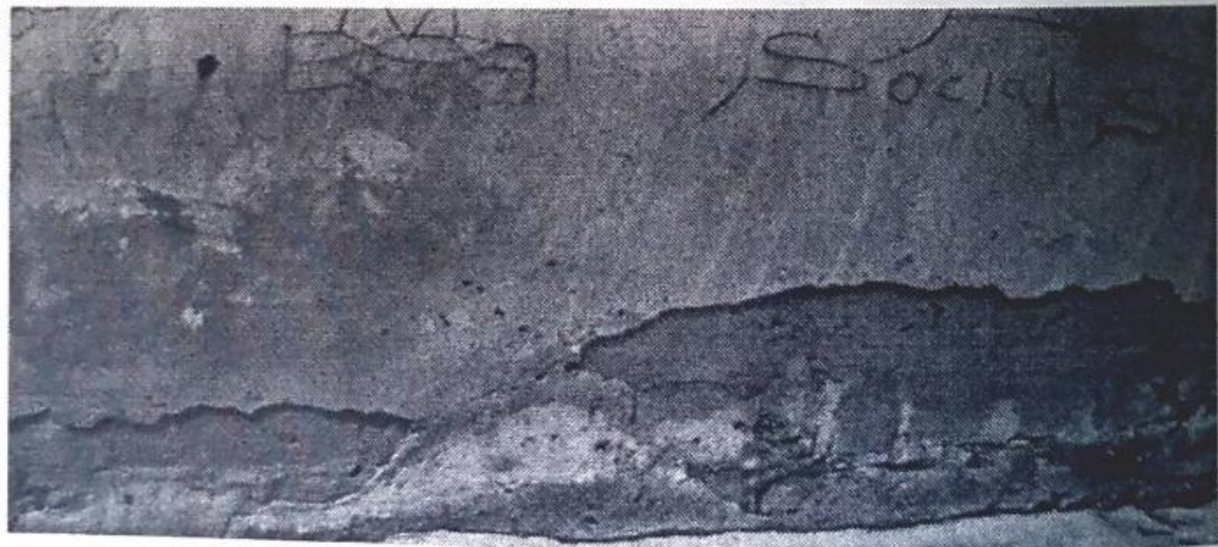
Figure 4. Severely Damped foundation and block walls.
