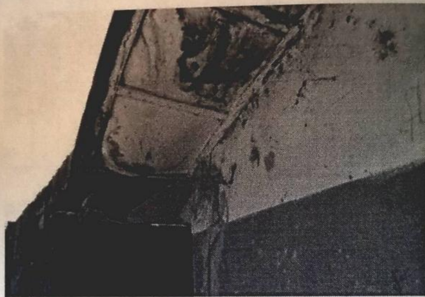
Figure 3. Damped facial board, ceiling and joist member.
