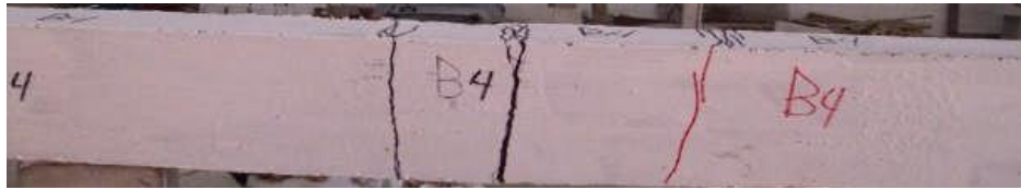
Plate I: Early first crack at mid-span of Beam 4
