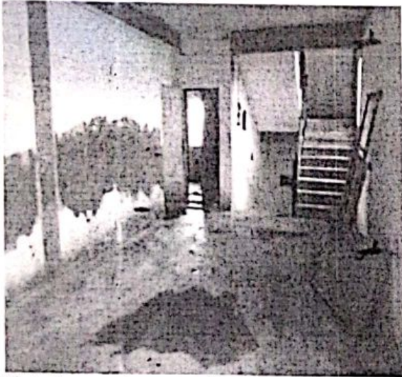
Plate 3: emergency stairs way of Male Hostel F.U.T Minna Gidan Kwano Campus Source: field work (2015)
