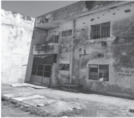
Plate 4.1: Students' accommodation in Alarming Condition
