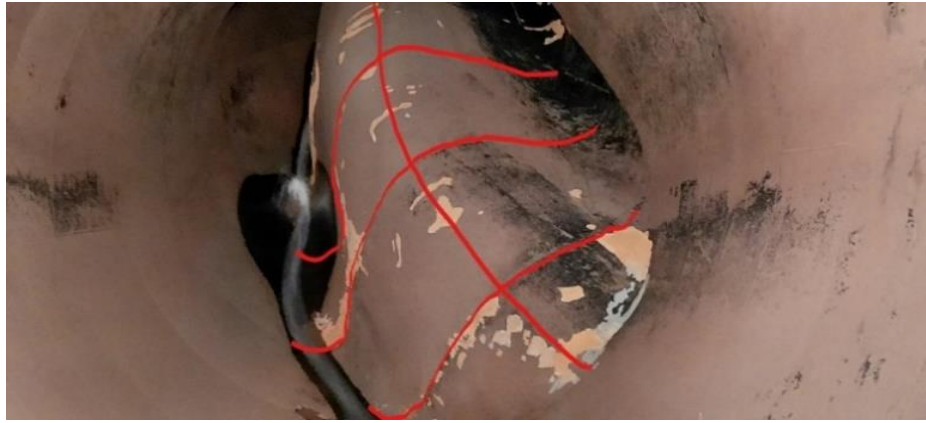
Figure 1.1: Buckling of underground Penstock (SHEP, 2020).
