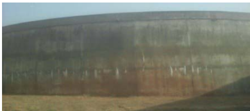
Plate IV. A clear water storage reservoir
