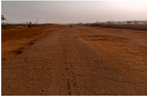
(c) Pavement surface with depressions
