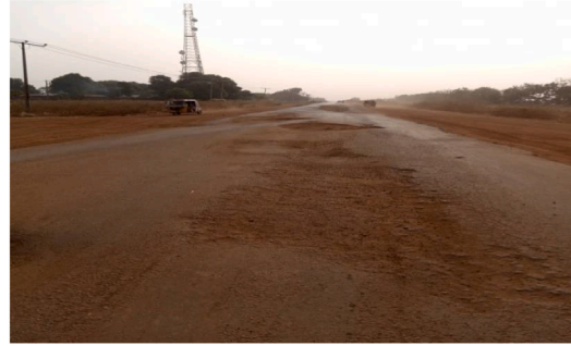
(b) Rough surface with wide potholes
