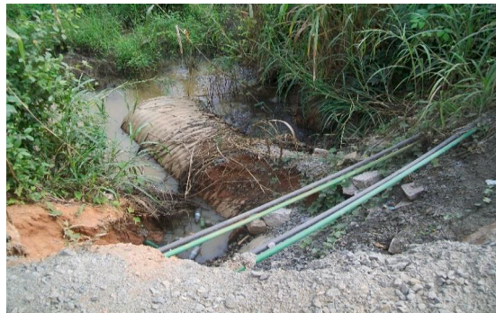
Fig. 5. Hollow metal sheet as water channel.
