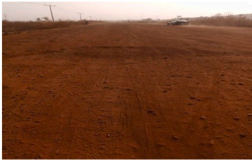
(a) Stripped asphalt surface with depression
