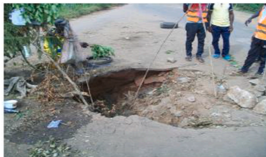
Fig. 6. Pavement failure over the embankment.
