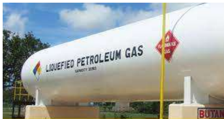
Figure 5: Liquefied Petroleum Gas Tank [13]
