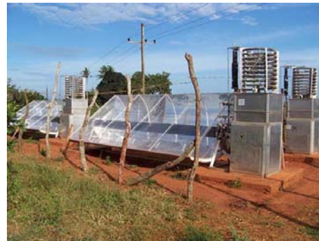
Fig 3: Three units were installed in Gwada District at Shiroro Dairy
