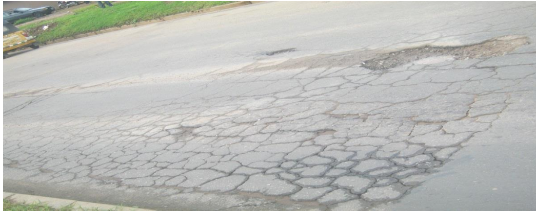
Figure1 A failed portion of the studied road
