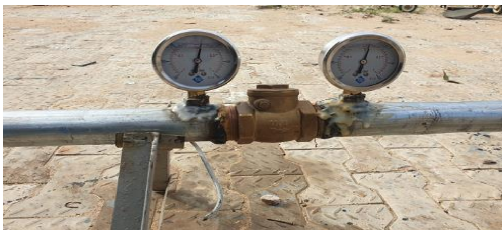
Plate III: Pressure gauges on the experimental test rig
