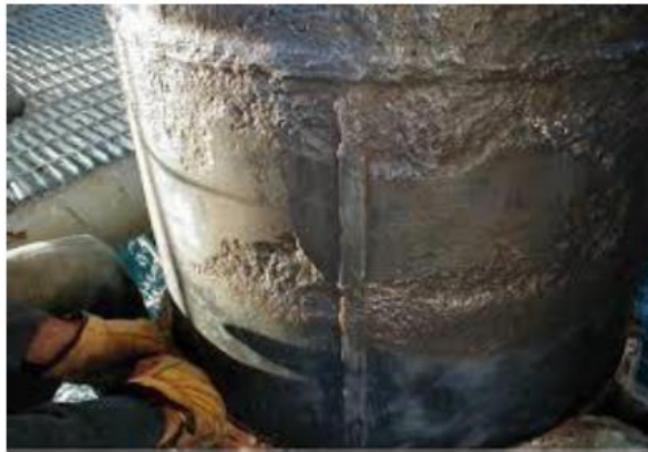
Figure 2.8: External corrosion in pipeline (Kalantzis, 2014)
