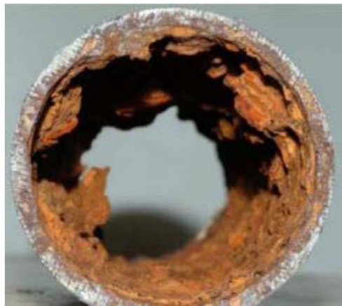
Figure 2.7: Microbial induced corrosion (Kalantzis, 2014)
