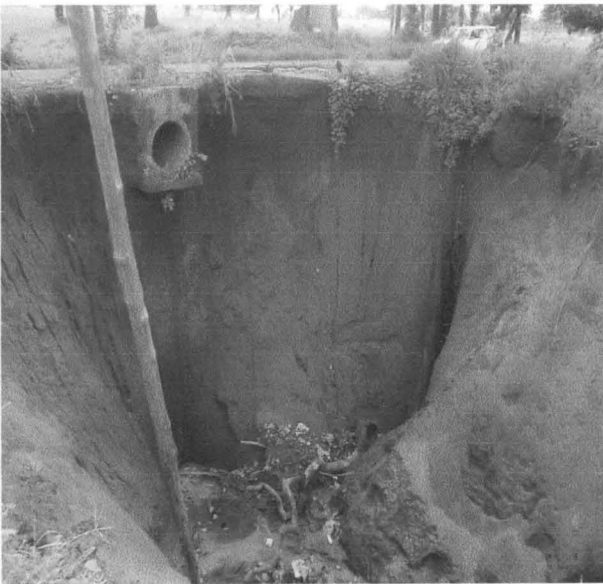
Plate iii: Menace of Gully Erosion Opposite C.O.E. Ankpa (L3)
