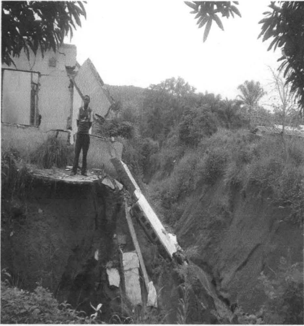
Plate v: Destructive effect of gully erosion on Structures opposite Chairman Quarters, Akpa (L5)
