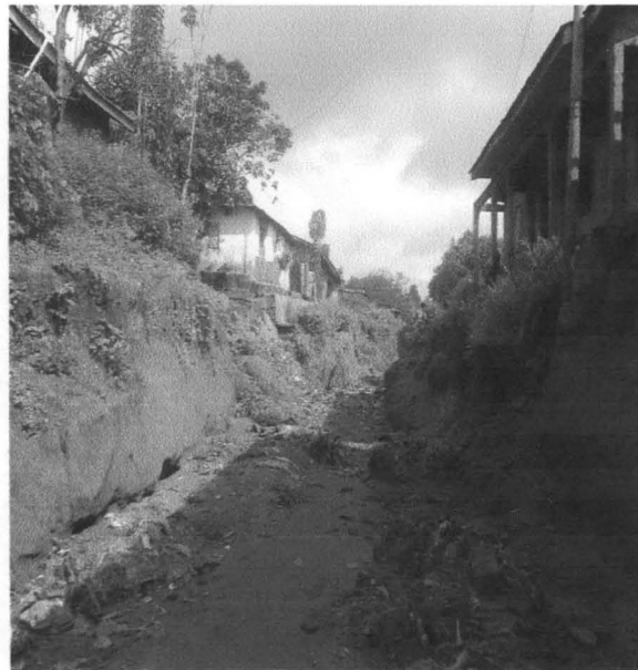
Plate iv: Gully Erosion at Ogwuchekpo Street, Ankpa. (L4)
