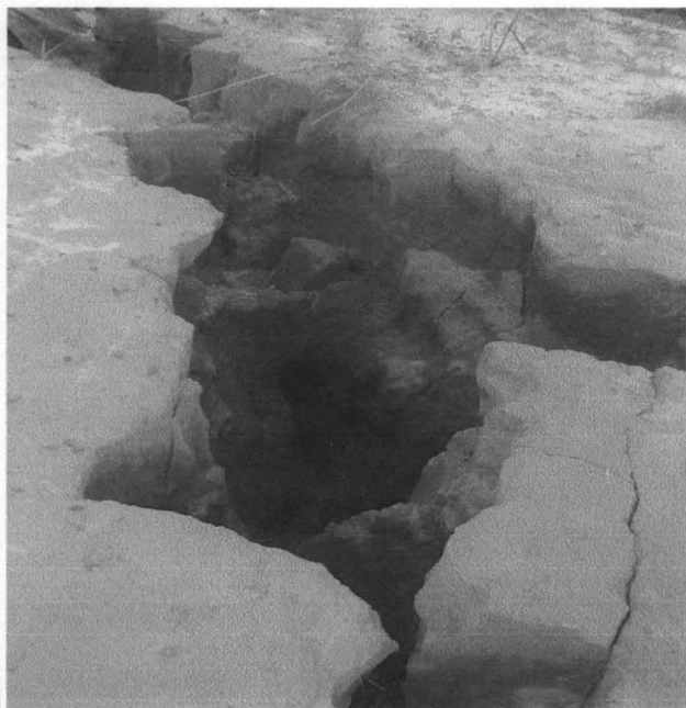
Plate xi: Gully erosion Opposite Community Sec Sch. Enjema Ankpa(L11)
