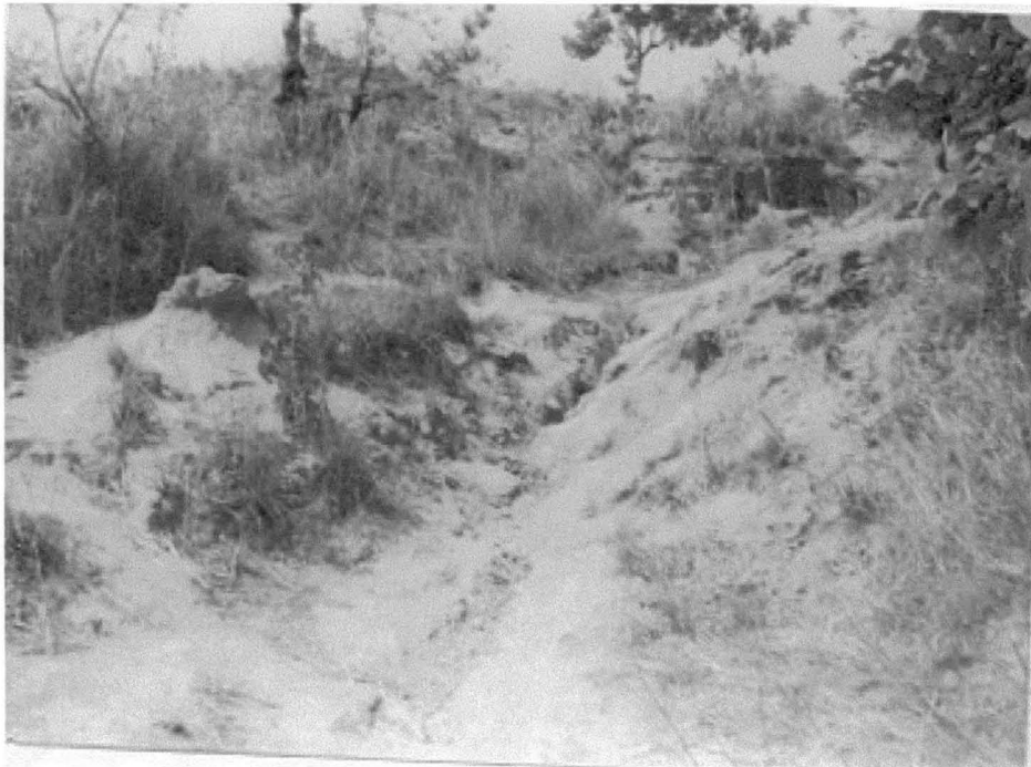
PLATE 13(b): This erosional activities has eroded over 20 metres length of the bank of the stream.
