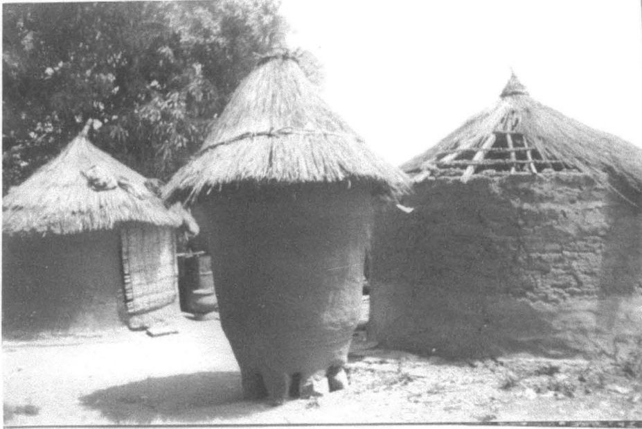
PLATE 1: SHOWING EFFECT ON ROOF WALL AND FLOOR
