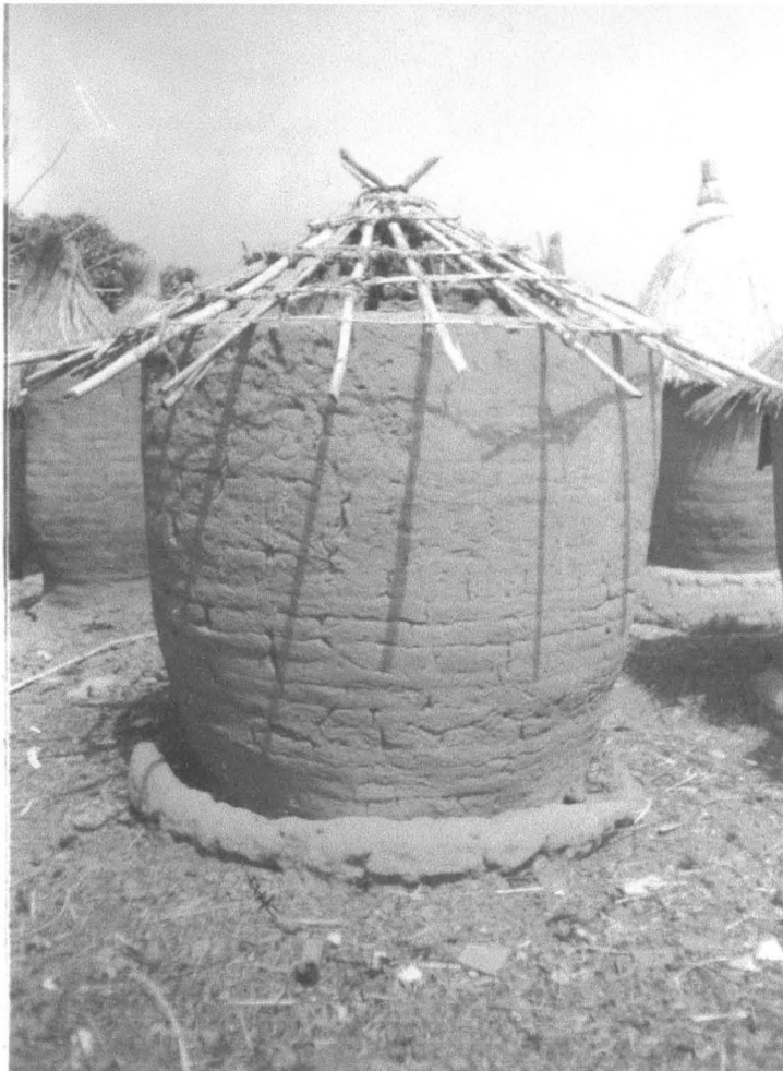
PLATE 2: SHOWING EFFEC ON FOUNDATION, WALL AND ROOF CONSTRUCTION
