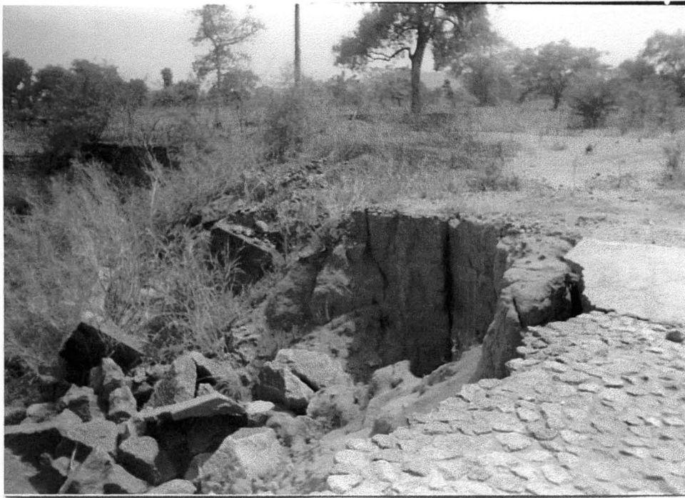
Plate 3 Picture Showing Erosion Effect due to the Impact of Construction
