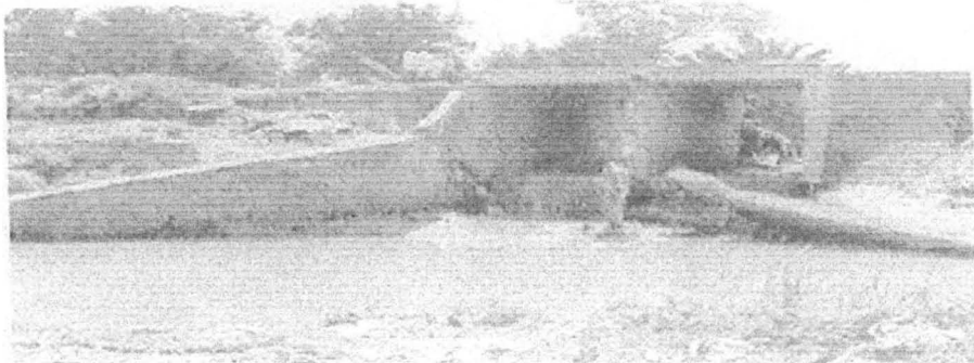
4.2.3: The above shows the hungry way in which we carelessly construct drainage, which lead to its subsequent collapsing and blocking the natural water ways, or inhibiting the smooth flow of water leading to flood and erosion in the urban city centres or towns
