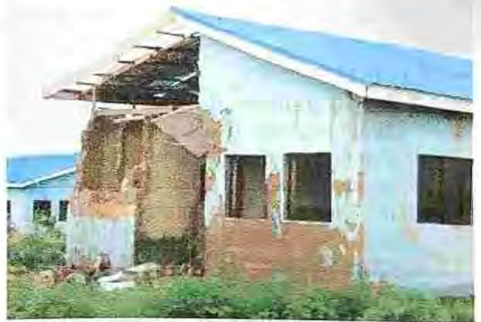
Plate 2 showing a structural failure of wall in 2 bedroom : Source authors' field survey 2010
