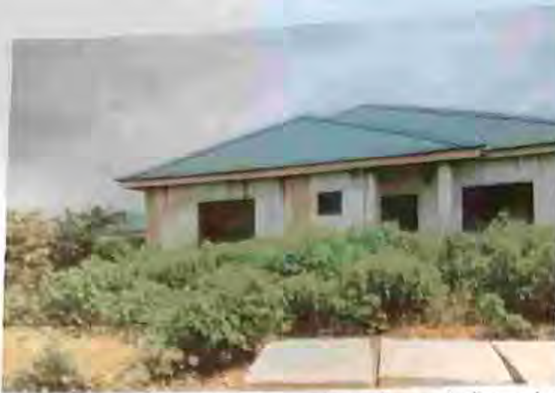
Plate 7. showing the outline of the column frames before painting was carried out. Source authors' field survey 2011
