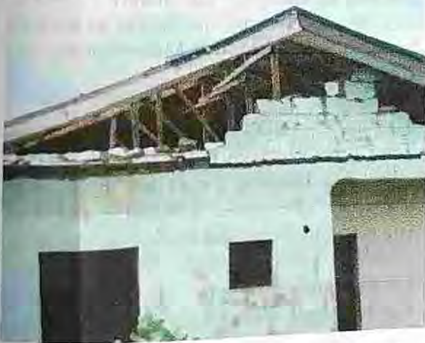
Plate 1; showing structural failures on the walls of 2 bedrooms. Source authors' field survey 2010
