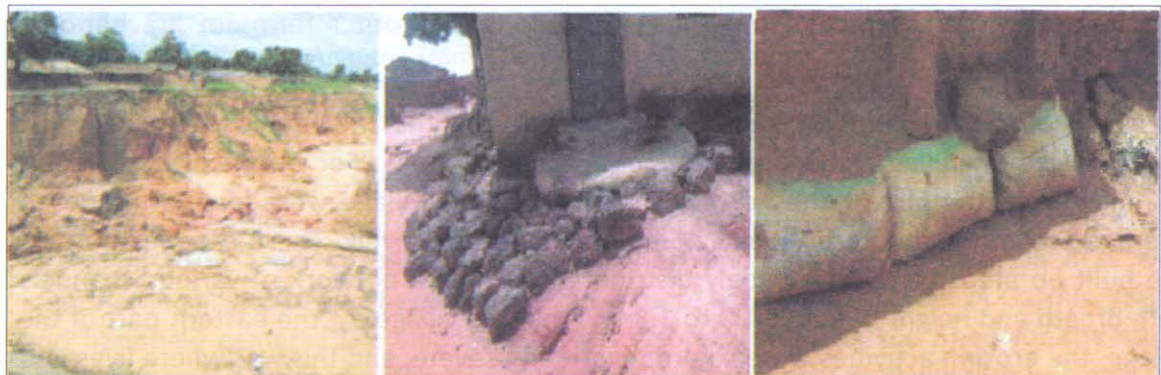
Figure 3. Gully erosion and sandstone used as foundation embankments in Rafingora.
