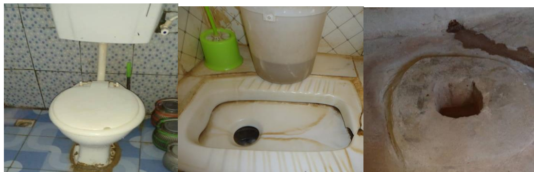
Plate 1,2 and 3: Water closet, pour-flush and pit latrine types of sanitation facility
