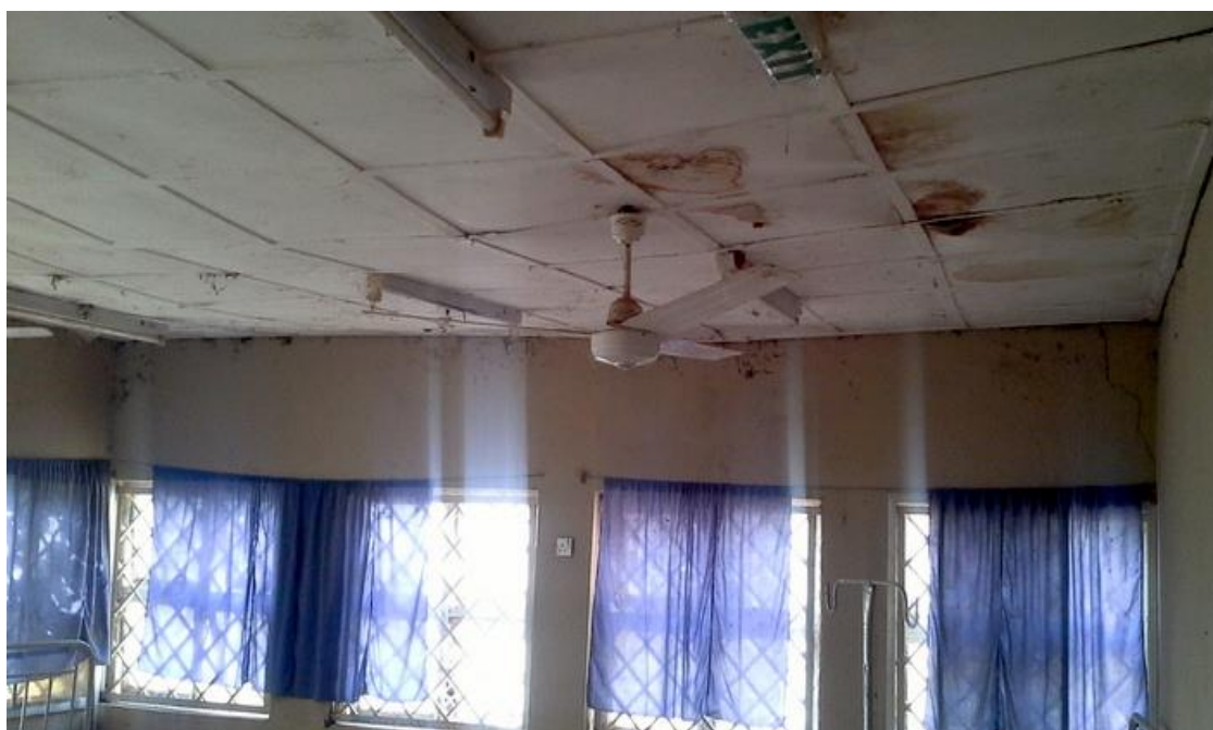
Plate I: Evidence of Leaking Roof in One of The Selected Health Facilities
