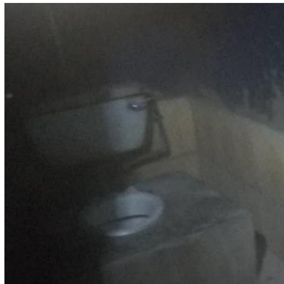
Plate V: Condition of Toilet Facility in One of The Selected Health Facilities
