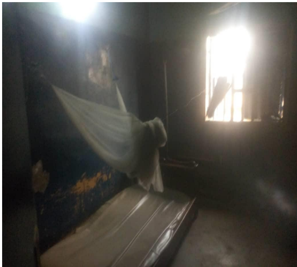
Figure 7: Evidence of Broken-Down Window in One of The Selected Health Facilities
