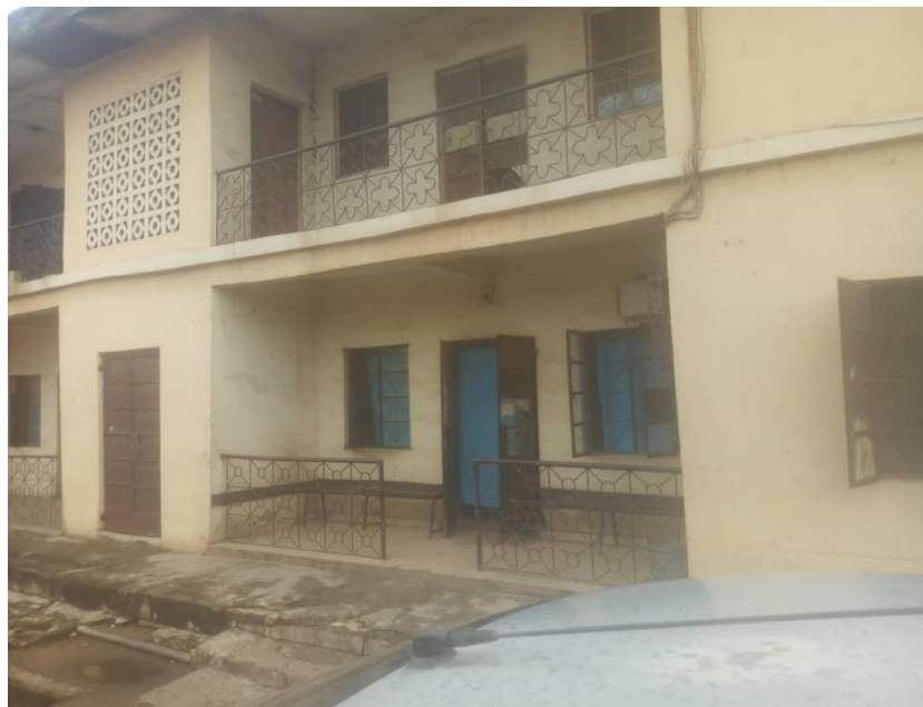
Plate III: Evidence of Worn-Out Painting in One of The Selected Health Facilities
