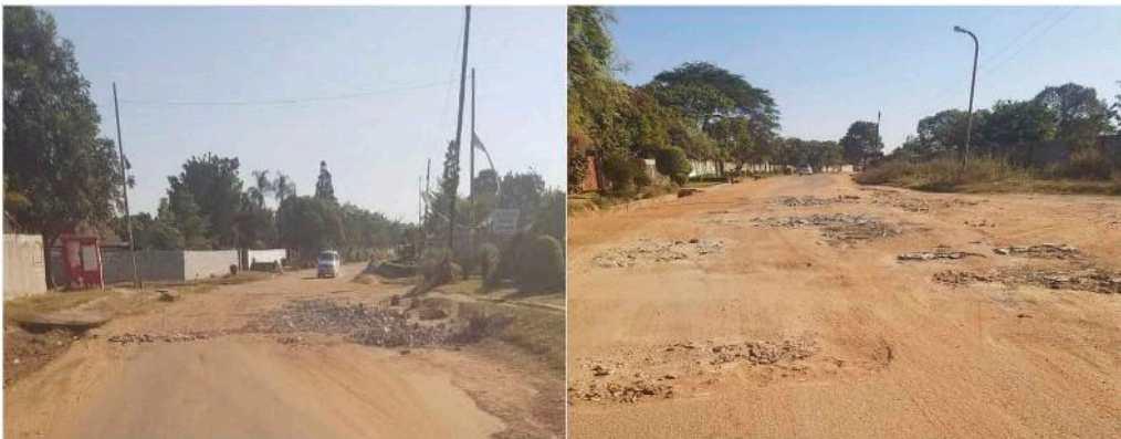
Figure 1. Concrete block debris used to fill potholes on Zambezi Road, Riverside, Kitwe.
