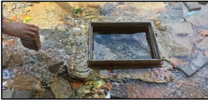
Figure 5. Leaking water valve, source, author's (2022).
