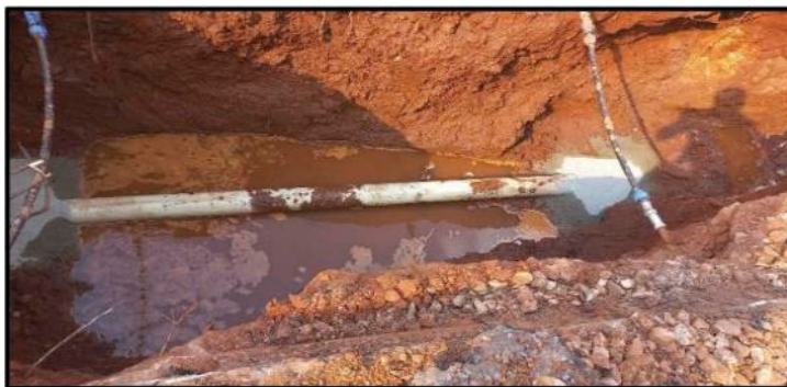
Figure 4. Broken water pipe. source, author's (2022).
