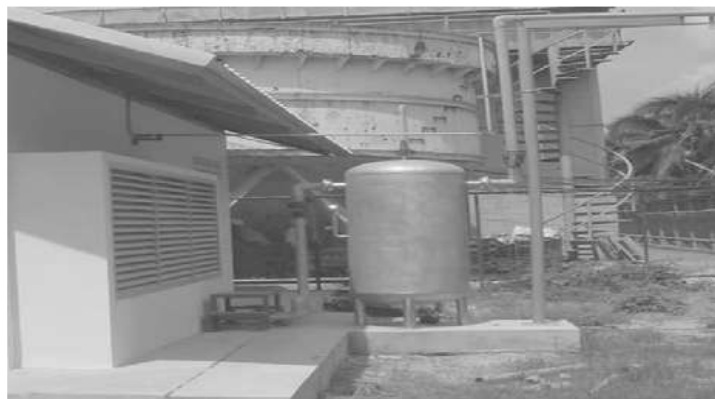
Figure 2.2: Biogas plant in Nigeria for the treatment of abattoir wastes from Bodija market, Ibadan. Source (Cows to Kilowatts, 2005)
