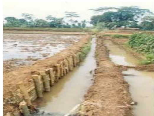
Plate 4: Mixture of rice straw and earth aterials used as lining for irrigation canals.
