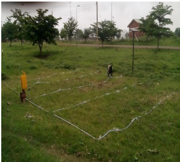
Plate 5: The side view of the drip system
