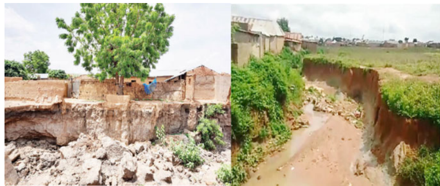
Fig. 2 An active erosion in northern, Nigeria
