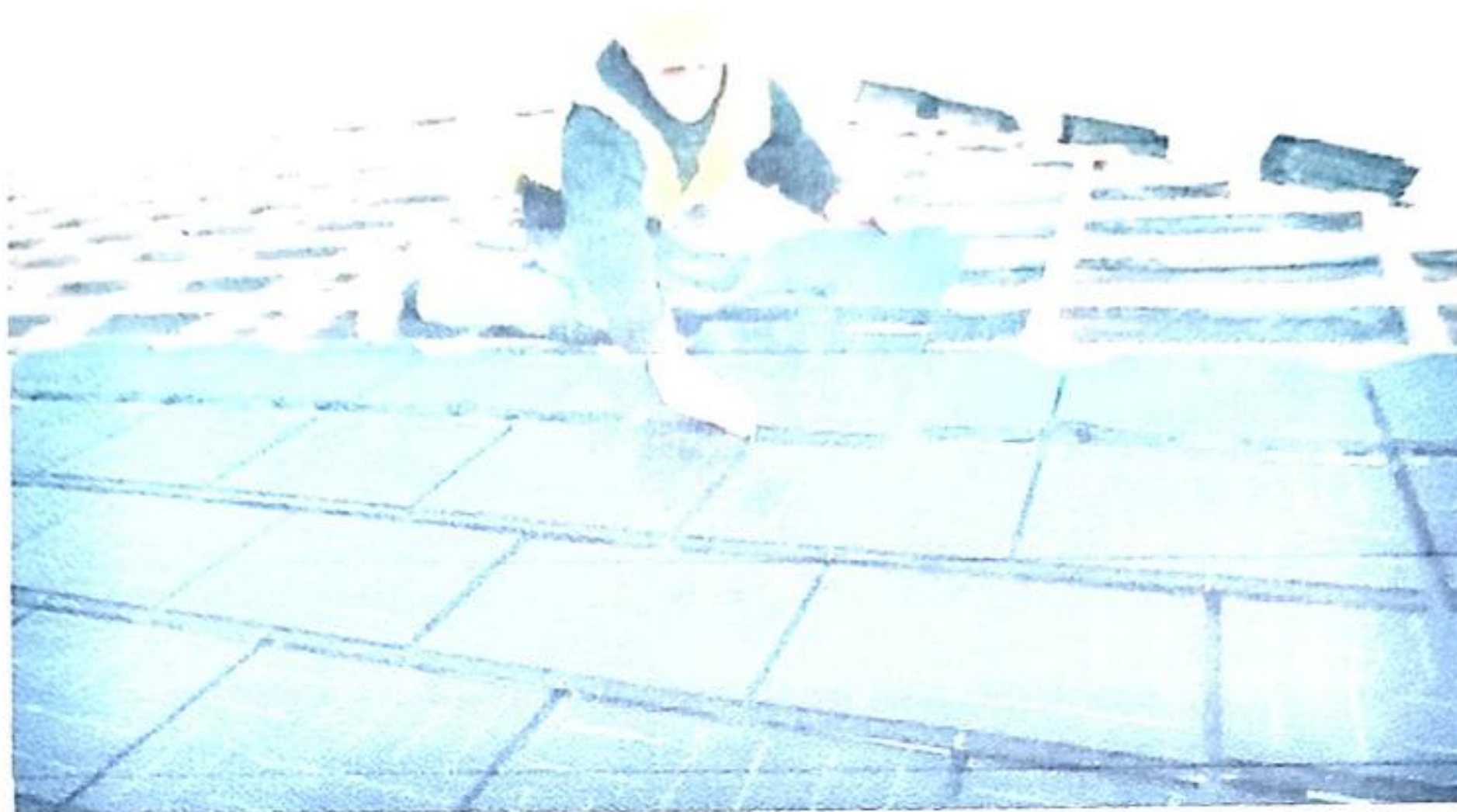
Plate 1: Photovoltaic cells used as roof cover for the building. Source Lyons (2007)
