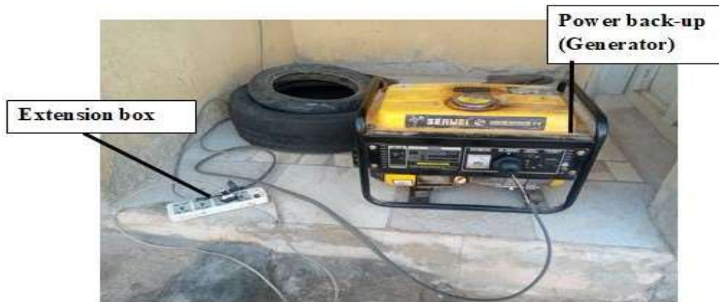
Plate II: Back-up Power Source
