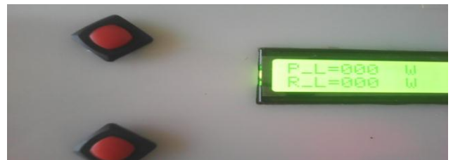
PLATE II: RESULT SHOWING THE CIRCUIT BREAKER READY TO BE PROGRAMMED TO DESIRED VALUES AND THE TWO BUTTONS USED TO PROGRAM IT.
