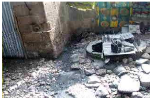
Figure 2: Affected Well Close to a Residential Toilet
