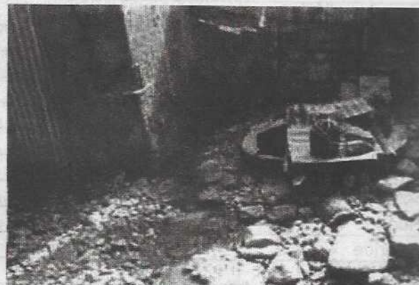
Plate 4.2 Affected well close to a residential toilet
