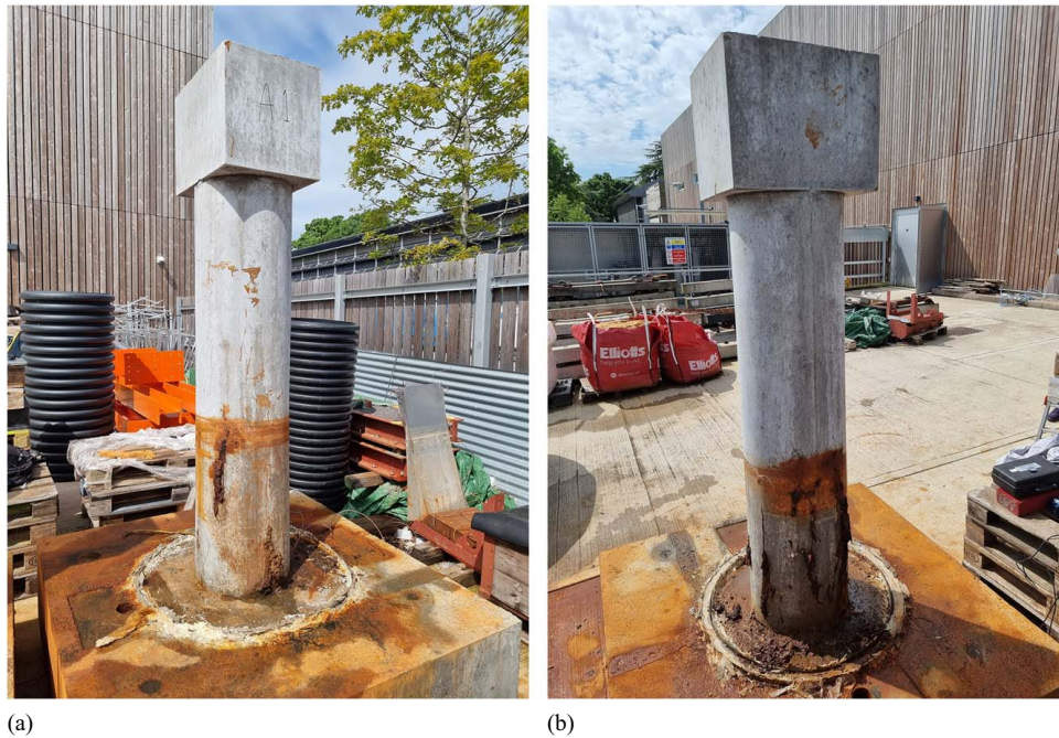
Fig. 3. Corroded columns: (a) Column A1; and (b) Column B1.
