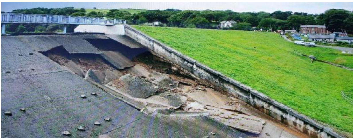
Figure 2 Collapsed Dam Whaley Bridge Dam in high peak (Duncan Leatherdale, BBC News, 2019)
