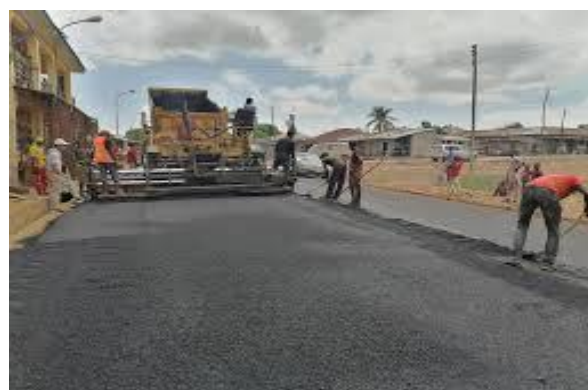
Figure 7 Asphalt Pavement of Emirs' Road Kaiama Round About, Patigi
