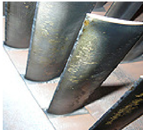
Figure 4. Compressor blades before cleaning
